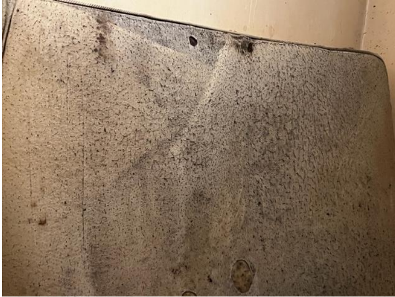
A mattress, black with mould, is leaned against a damp exterior wall in a bedroom.
