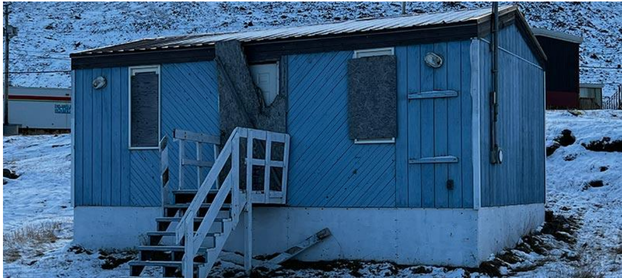
A house sits boarded up waiting for repairs.
