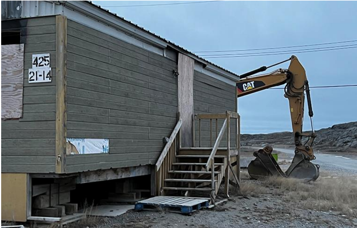
Home in need of repairs in Rankin Inlet.
