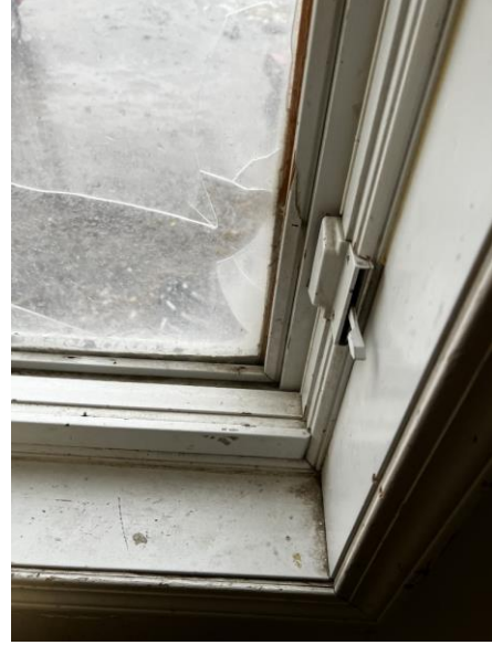
Low quality window hardware.
