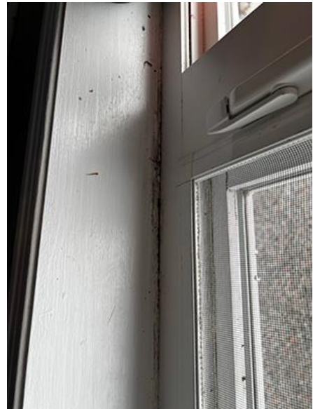
The window casings throughout this house show damage from condensation and black mould from sitting moisture.
