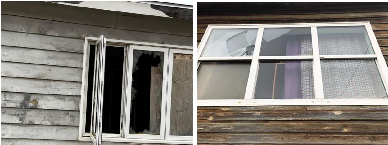
Broken windows, as well as warped window and door frames, allow heat to escape, driving up heating costs.
