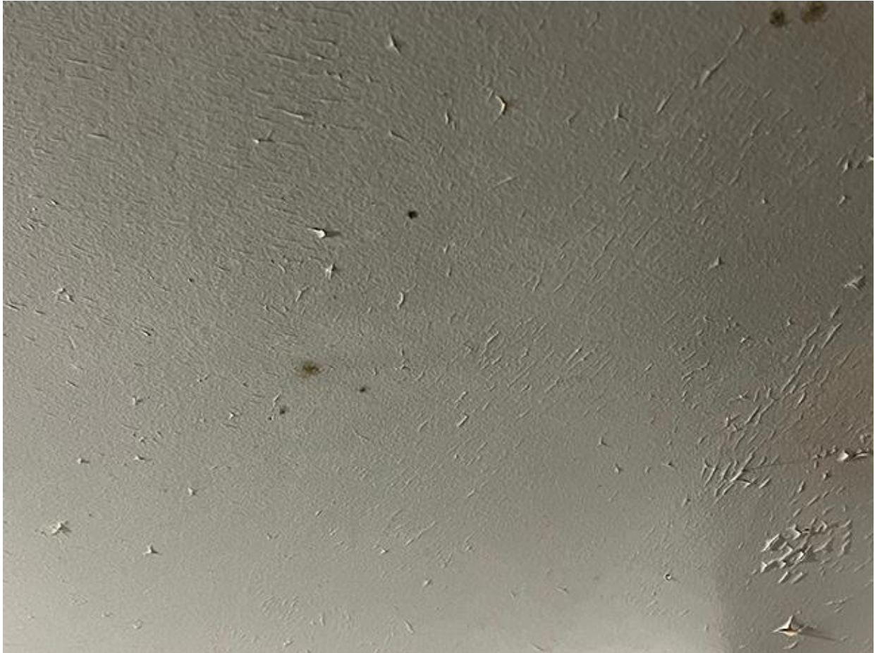
Signs of mould in bathroom in Pang.
