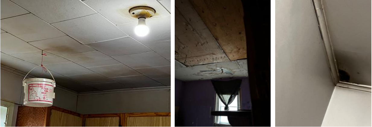
Water staining and likely black mould covers the ceiling in multiple houses.
