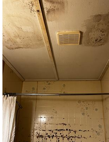
A bathroom shows obvious signs of water damage and mould.
