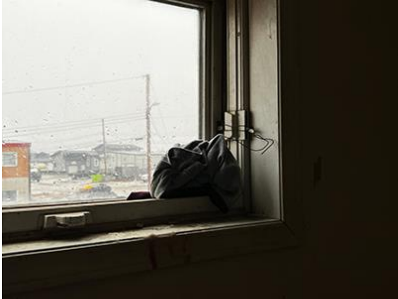
Rankin Inlet: Clothes stuffed in a broken window to retain heat.
