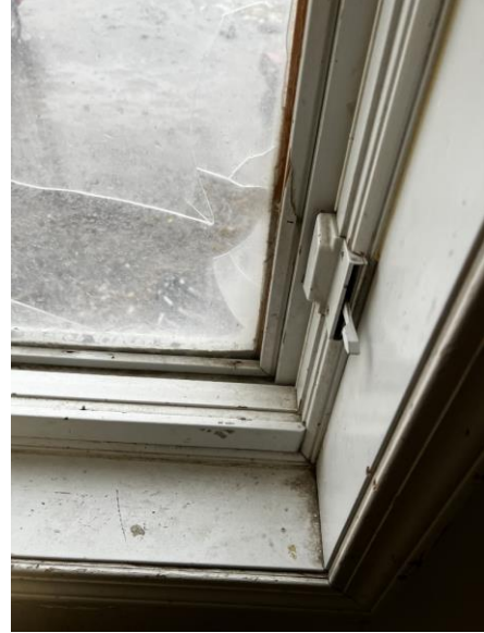
Low quality window hardware.
