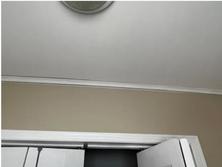
A gap in a new house has begun to appear where the ceiling is bowing away from the wall.
